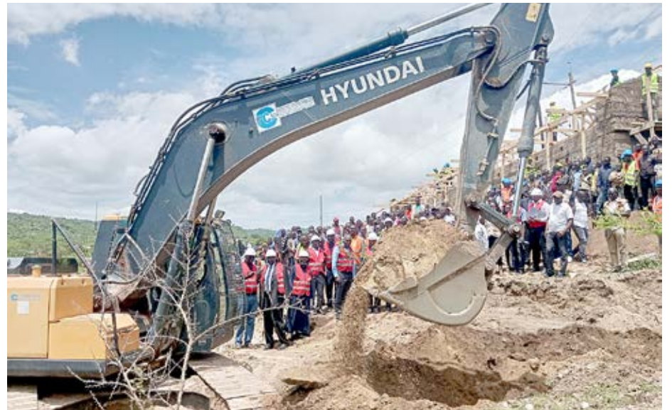
Water Principal Secretary Julius Korir during groundbreaking ceremony for the Mtembur-Kitalakapel project in Kapenguria Constituency.
