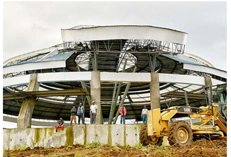
The Modern Fish market under construction in Karai area along the Nakuru-Nairobi Highway. Its set to revolutionize fish production and marketing in the Lakeside town of Naivasha.
