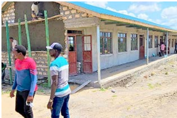
Classrooms under construction at Burangi Primary School, Malindi Sub-County funded by MISHDP II. Photo by Haniel Mengistu.
