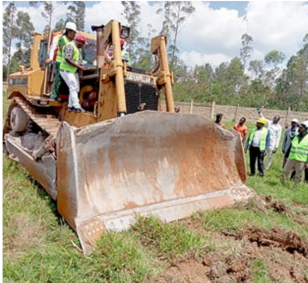
Mining, Blue Economy and Maritime Affairs Cabinet Secretary (CS), Salim Mvurya accompanied by Kakamega county leaders, senior government officials and contractors awarded the construction of a Sh5.8 billion gold refinery at Lidambitsa area, Ikolomani constituency of Kakamega County. PHOTO: GEORGE KAIGA.
