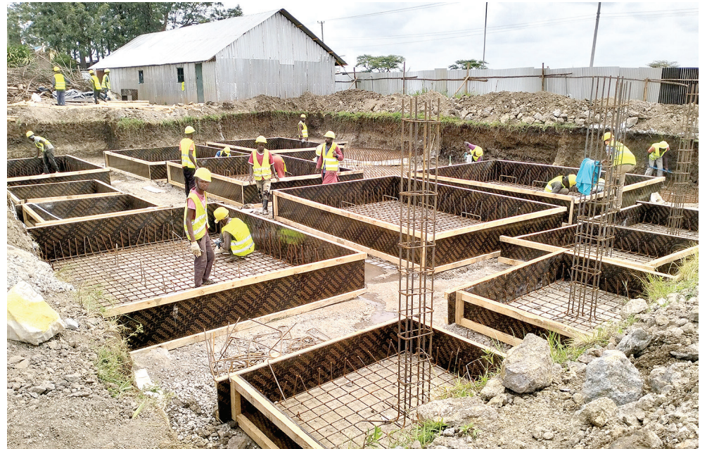
Construction of affordable houses at Makenji area in Kandara constituency, Murang'a going on
