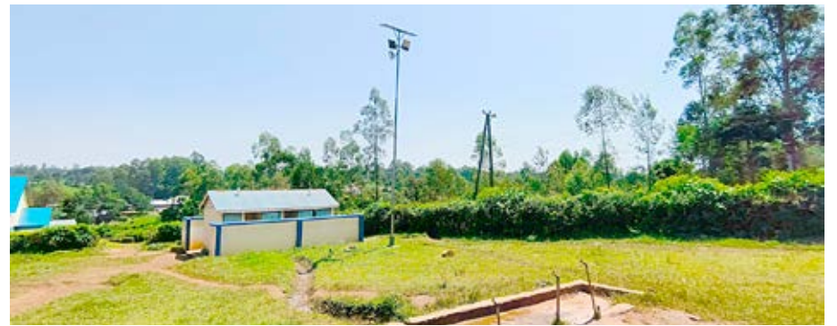
A high mast floodlight was installed at Mwhila Boys high school in Khwisero Kakamega to provide security lights to the school. Photo by Moses Wekesa.
