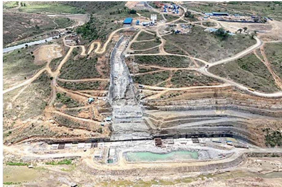
An aerial view of the ongoing construction of the multi-billion Mwache dam in Kinango Sub-County, Kwale. PHOTO: ANDREW HINGA/KNA
