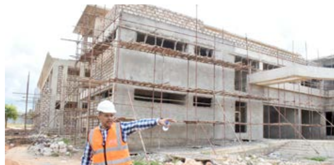
A team from the Ministry of Education and Inter-University Council for East Africa (IUCEA) inspects construction works at the Regional Flagship Marine Transport and Logistics Centre in Kwale County.
