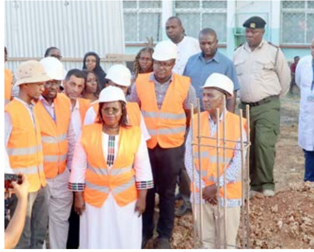
CS Peninah Malonza (Second Right) accompanied by PS Kello Harsama (Right) inspects the construction of the ICU facility at the Malindi Sub-County Hospital.
