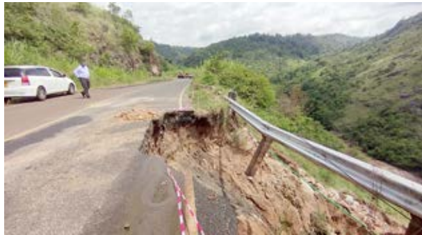
A section of the Murang'a – Kiriaini road that was destroyed by Mudslide last week.
