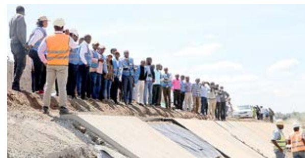
Officials from National Irrigation Authority join the PS Irrigation in inspection of ongoing canal construction.
