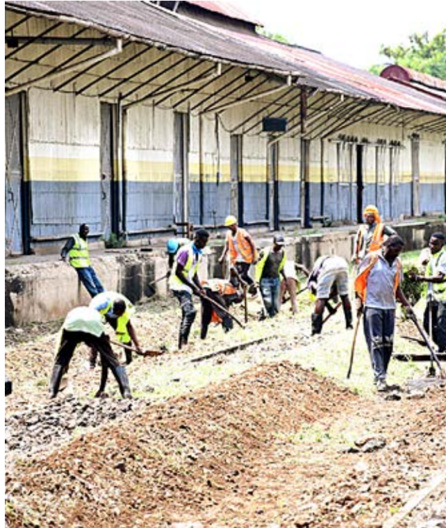
Rehabilitation of the Meter Gauge Railway going on at the Mombasa Central Railway Station. PHOTOS: CYZICK SIDAYI
