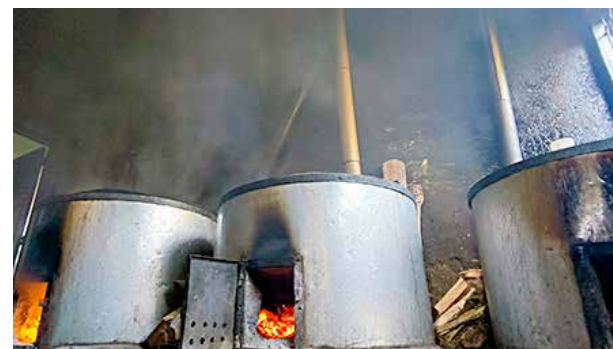
A kitchen at a school in Kakamega. Smoke emanating from the firewood discolors walls and floors.
