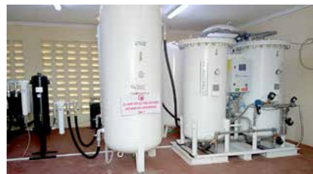
Oxygen Plant in TransMara west Sub County Level 4 Hospital
