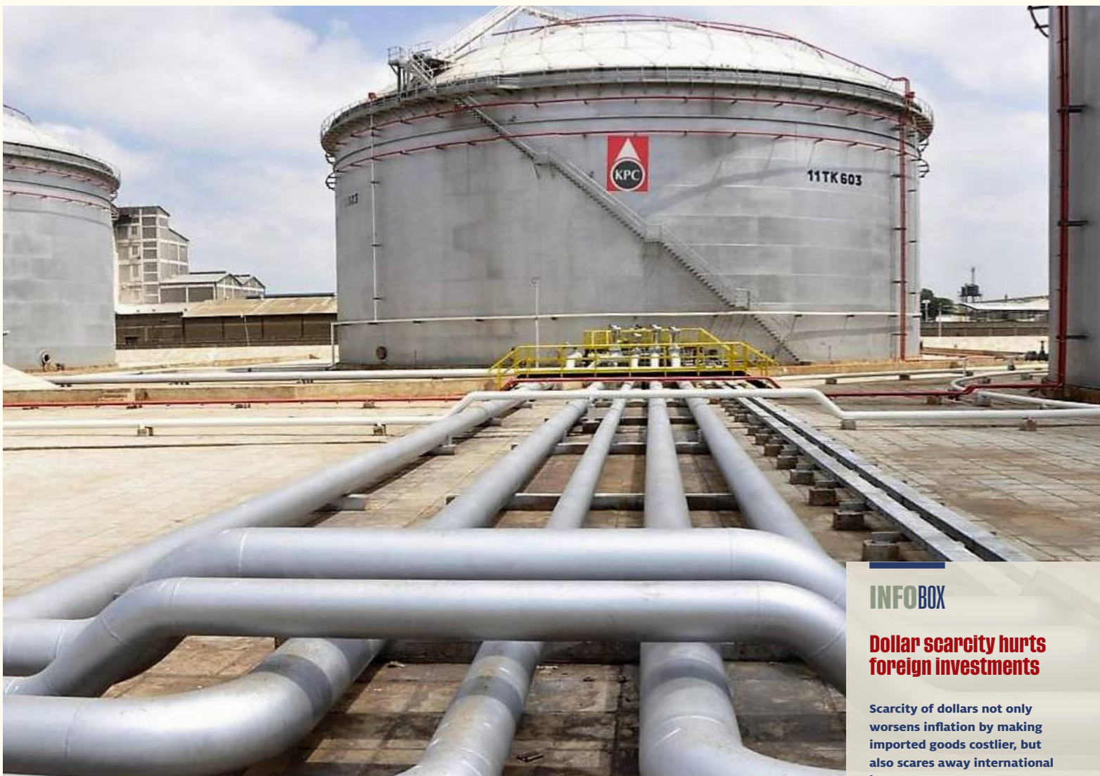
A Kenya Pipeline Company depot. Kenya will import its monthly fuel needs from two government firms in the Gulf.
