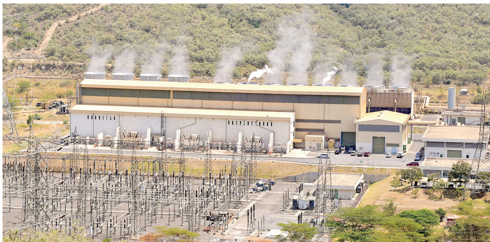
A geothermal power plant located at KenGen Olkaria wells in Naivasha. KenGen has earmarked 4,000 acres near the power plants where investors are set to establish industries powered by steady, cheaper geothermal power. PHOTO: ERASTUS GICHOHI
