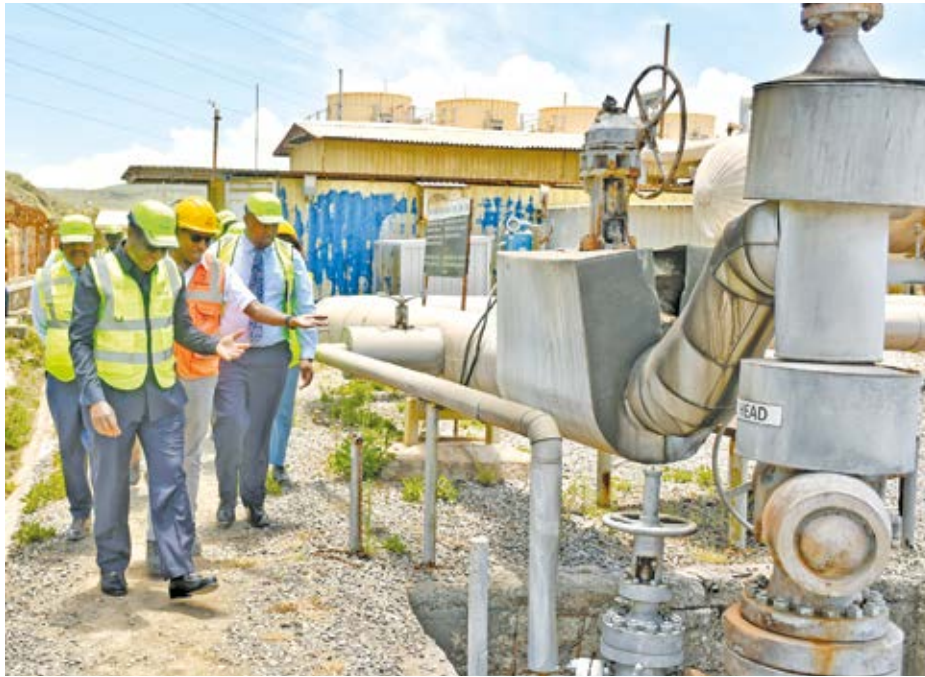
Energy and Petroleum Cabinet Secretary Hon. Opiyo Wandayi (left), joined by the ministry office, inspects a geothermal wellhead during his official familiarization tour of geothermal-rich Olkaria area in Naivasha. Photo by Erastus Gichohi.
