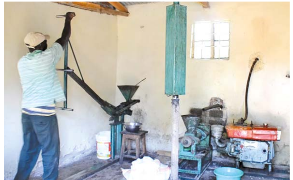
A small-scale sunflower oil processing plant at one of the farmers. Photo by Moses Wekesa, KNA.
