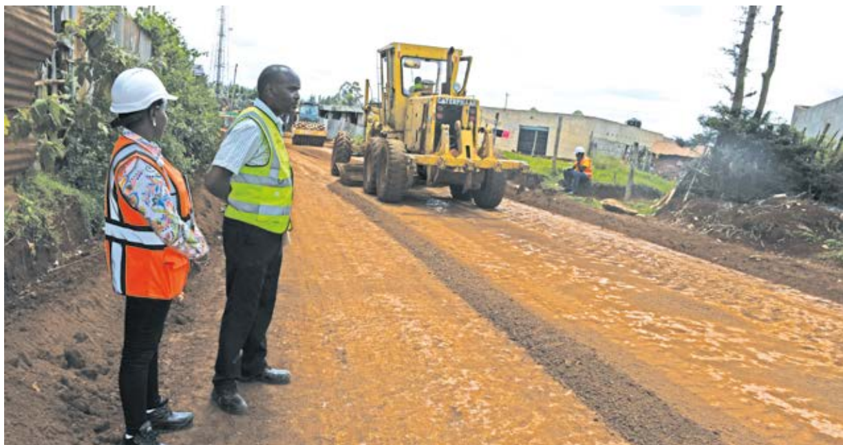
Jane Mwangi Nandi County KISIP 2 Project Assistant Resident Engineer during earthworks road in Mosoriot town.
