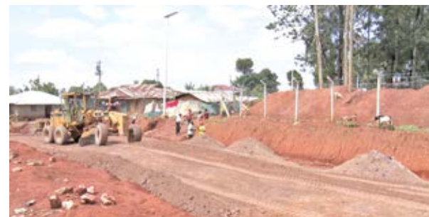
The ongoing road upgrade at the Amalemba Informal settlement in Kakamega Municipality through the Second Kenya Informal Settlements Improvement Project (KISIP 2). Photo by Moses Wekesa, KNA.
